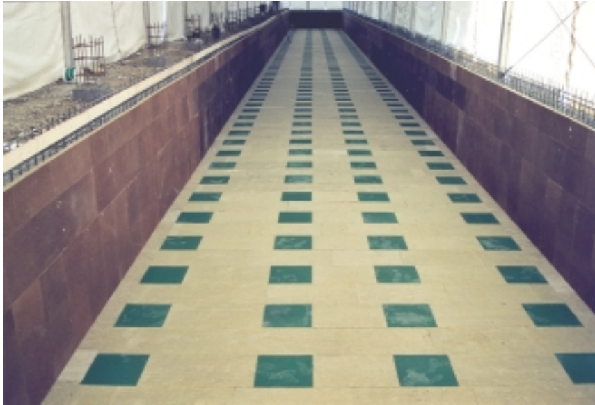
Figure 8: Foundation pit constructed with AirLoc isolation system for the reduction of vibration and structural disturbances
