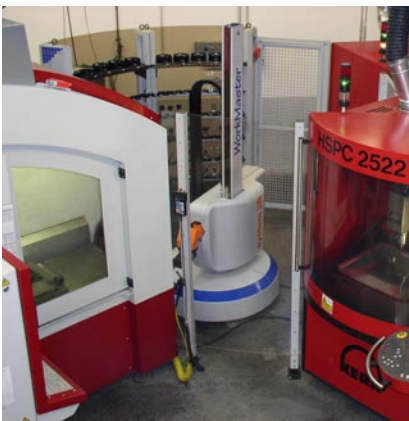
The triple cell at GKN, integrating 3 milling machines fed by the WorkMaster robot from System 3R.
